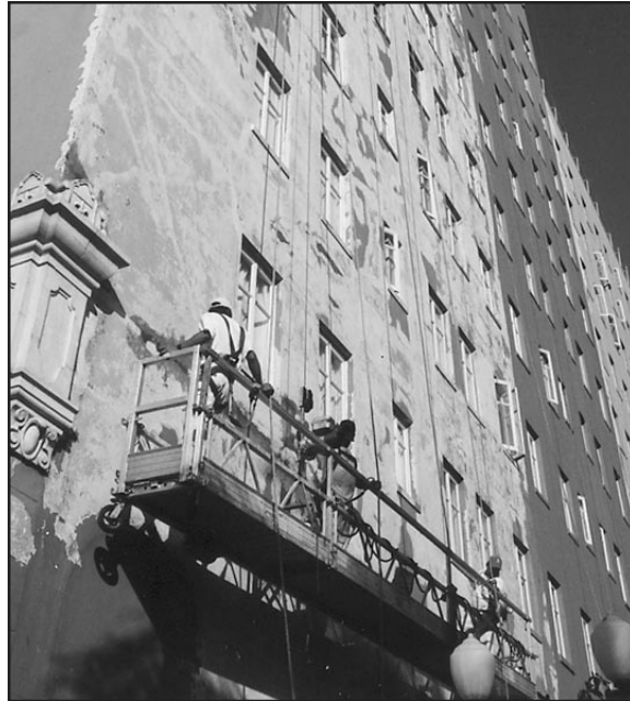
Men at work: scraping and sealing, patching and painting the Campbell building. The latest in a series of planned improvements to the Lafayette complex.
